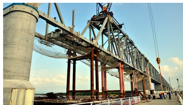
The Tong Jiang–Nizhnelenskoye “broken bridge” (Photo: World News01.com)
